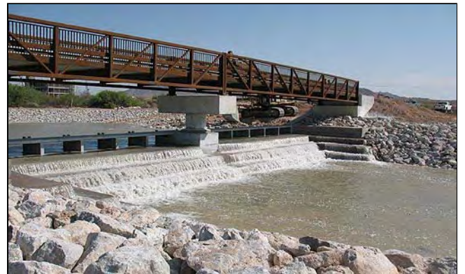
The eastern section of the bridge over the newly diverted bypass channel.
