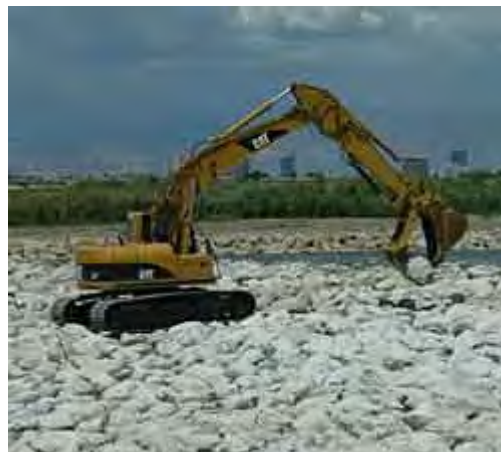
Construction crews work on the final details of the Ducks Unlimited No. 2 Weir.
